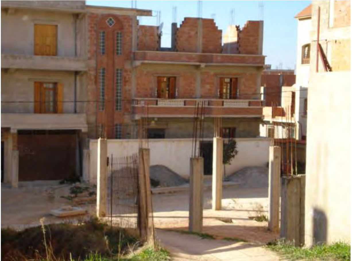
Figure 67: The lasting work in different locations of a housing development. Posts with steel bars coming out and facades with no coating characterize this built environment. This does not leave any coherence in the perception of the street scape. (author, 2008).
